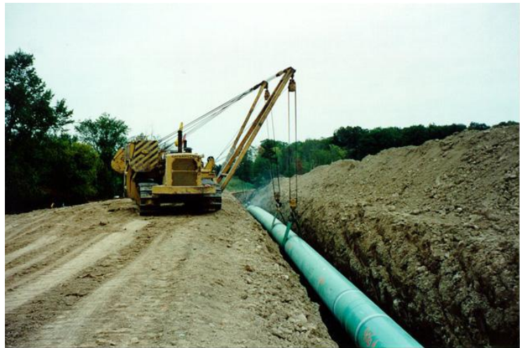
The gas crew is installing the last of the piping Courtesy FERC, image is in the public domain
