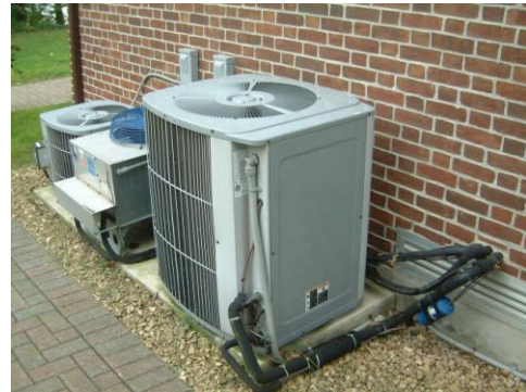
George’s crew has calculated the load for a new building AC unit Courtesy Achim Hering via Wikimediacommons, image licensed under Creative Commons
