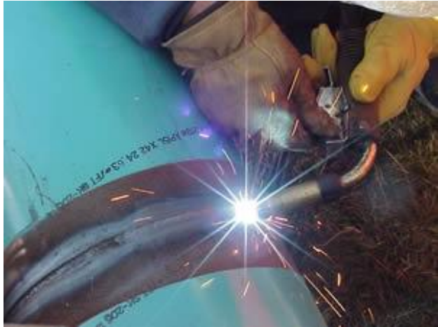
Roberto is welding new gas lines Courtesy U.S. DOT, image is in the public domain
